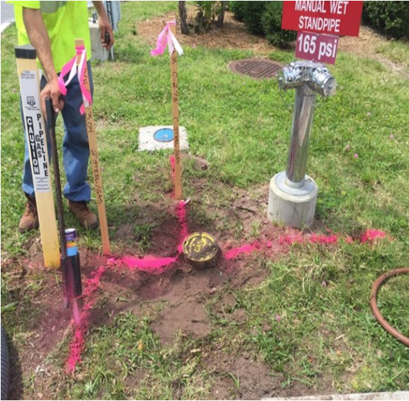
Figure 3: a natural gas valve that was previously buried and brought back to grade. The service lines are then located for campus map updates.
